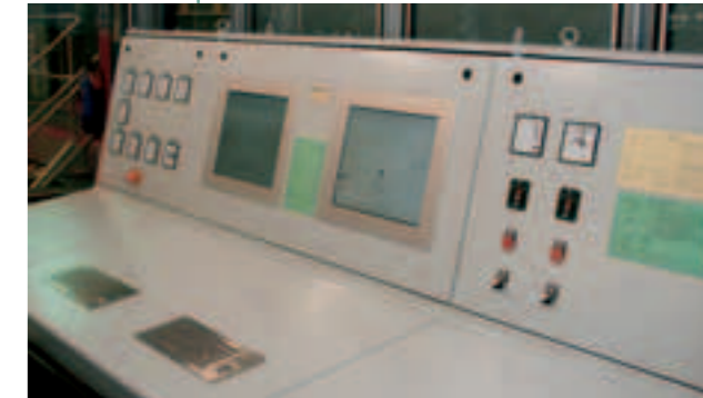
Plain control desk (Power Management System) in Stanley Power Station
